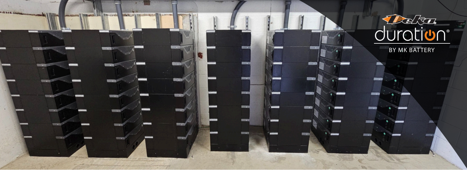
Battery Storage System — 56 DD5300 battery modules providing primary site power
